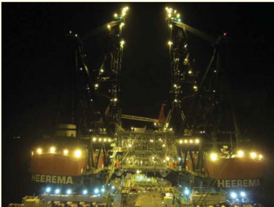
Shell Oil Co. recently completed installation of the drilling and production platform at its Perdido development in the Gulf of Mexico. Photo from Shell.
